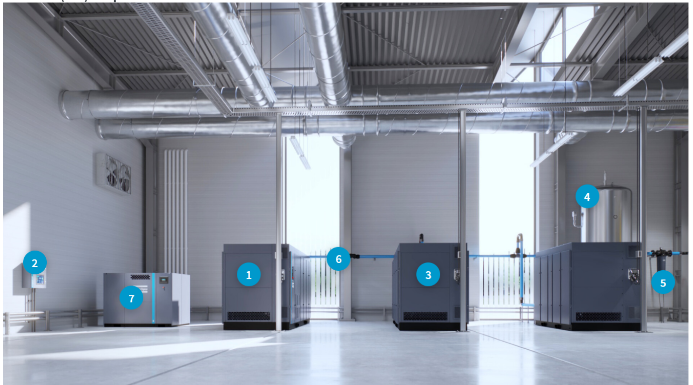
ZR 160-315 (VSD) Compressor Room Installation
